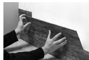
3) When placing tiles on the second row and beyond, angle the tile back about 30 degrees and rest the bottom edge on the tile below, then slide it over to butt the previous tile.
